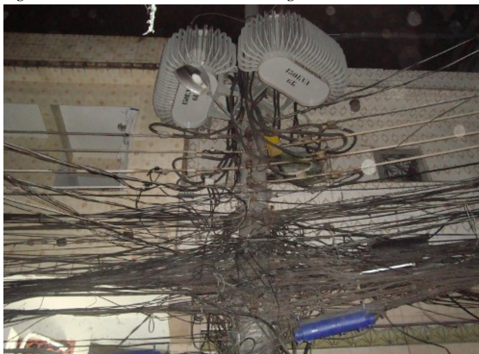
Figure 3. An electrical transformer in the Manguinhos district
